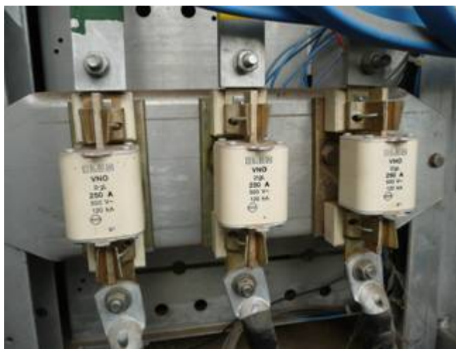
Electricity connections will need special metering equipment
